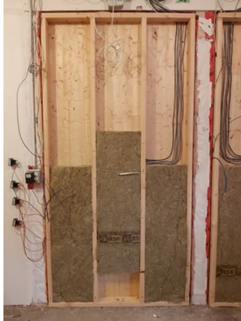
Figure 23. Stone wool batt insulation (nominal R14) installed to cover sensors installed from the interior surface of CLT.
