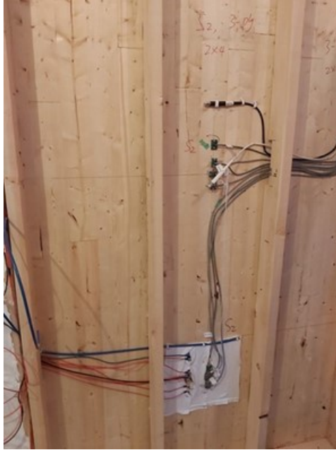
Figure 7. A photo to show the sensors (mid-height, bottom with the interior wetting pad) and wiring installed inside one wall panel (S2) with the interior service wall framed.
