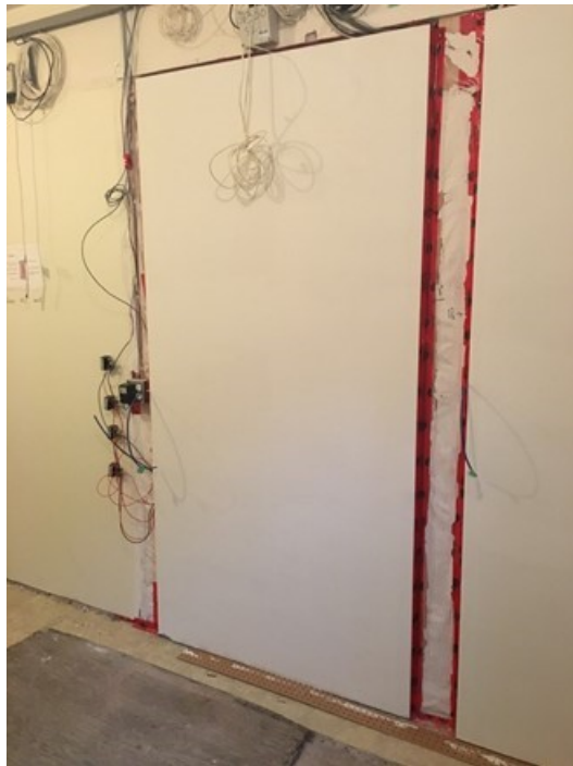
Figure 26. Each wall painted with a regular primer and two coats of top finishing.
