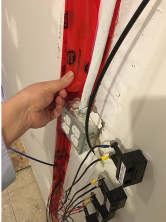
Figure 25. The edges (including those of drywall) of each wall sealed with a tape.
