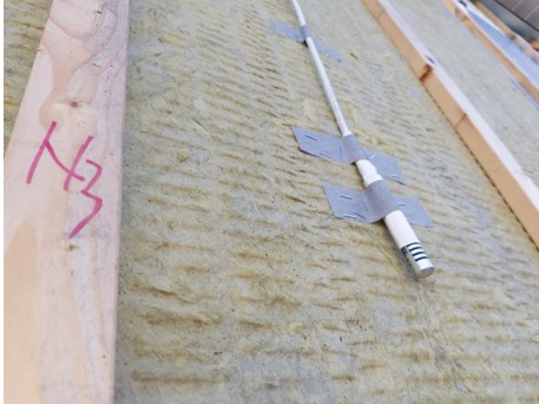
Figure 19. An RH/T sensor installed in the rainscreen cavity of each wall.
