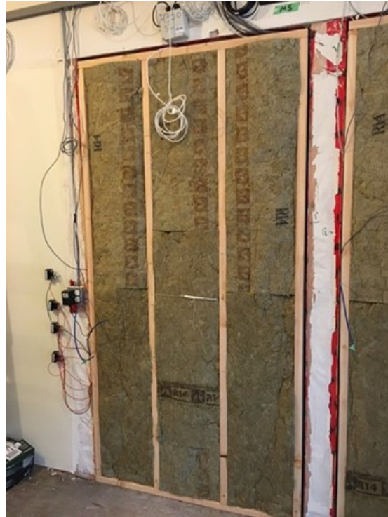
Figure 24. Stone wool batt insulation installed in the interior service wall cavities of walls No.1 and No. 2.
